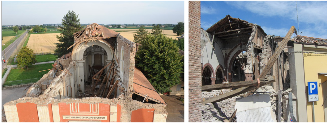
Fig. 1. San Martino, Buonacampa and San Francesco D'Assisi respectively, Emilia Romagna (Italy), damages after 2012-Earthquake.
