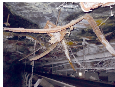
Fig. 3. Corroded mesh, channels, and roof bolts.
