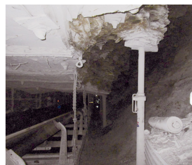
Fig. 4. Cutter roof failure.
