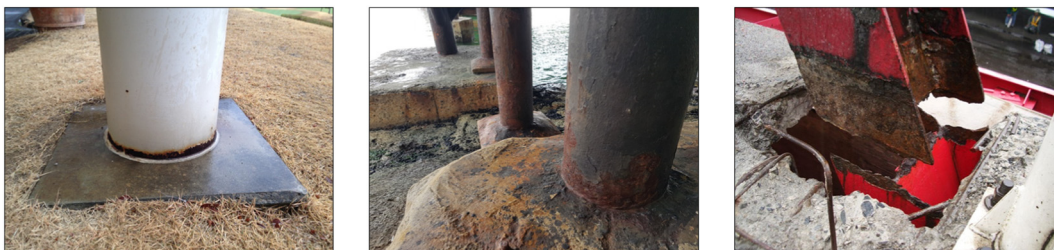
Fig. 3. Local corrosion at bottom ends of steel columns.
