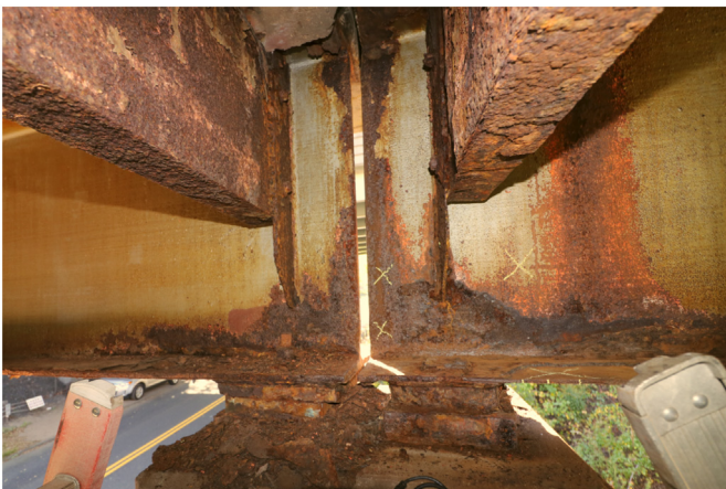
Fig. 2. Corrosion at girder end.
