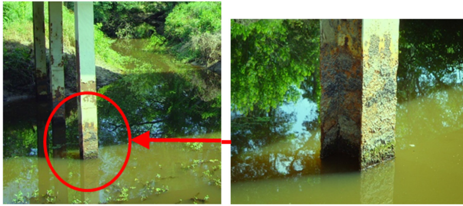
Fig. 1. Localized corrosion of H-piles from field visit.
