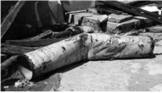
Fig. 1. Large plastic deformation at the pipeline section [1].
