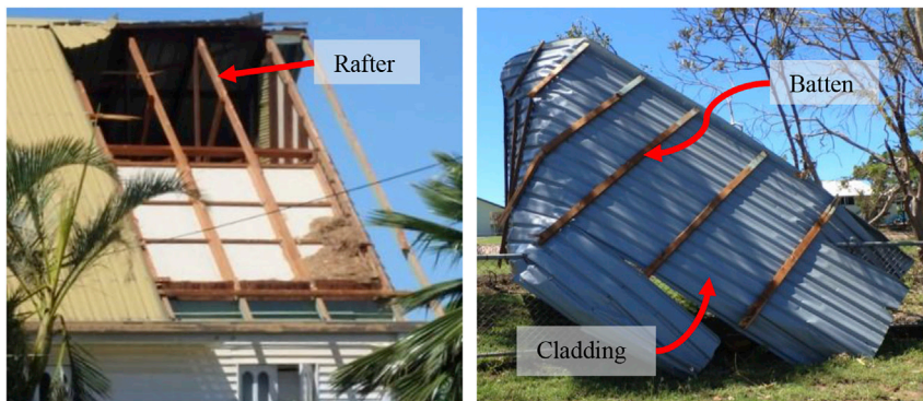
Fig. 1. Typical batten-rafter connection failure: large section of the roof envelope removed (right) with cladding still attached to battens and rafters left intact (left). Adapted from Boughton et al. (2017).
