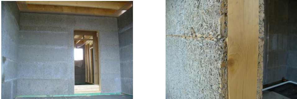
Fig. 1. (a) The usage of timber-cement boards as a wall-cladding - general view (b) detail
