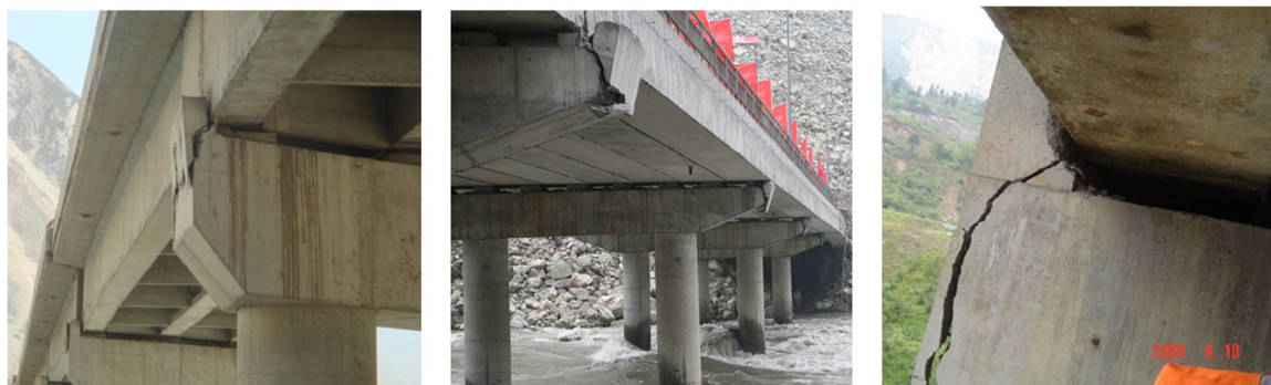
Fig. 1. Typical shear key damages during the Wenchuan earthquake (diagonal shear failure).
