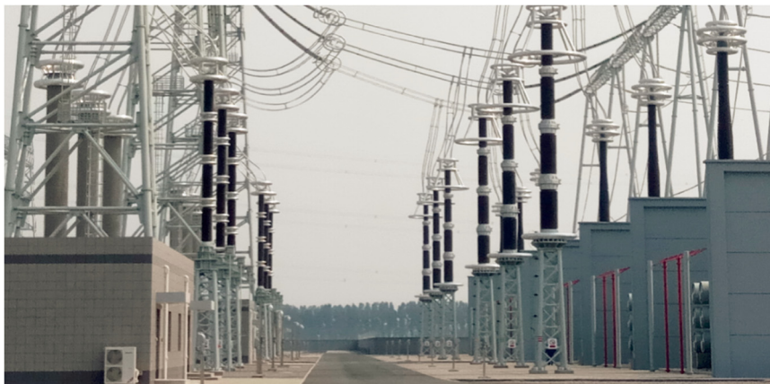
Fig. 3. Cylindrical electrical equipment in 1000 kV Beijing East Substation in Beijing, China.
