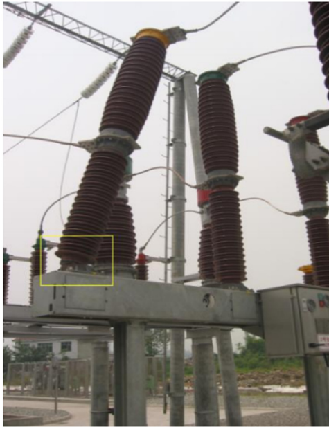
Fig. 1. Failure of cylindrical electrical equipment in 2008 Wenchuan Earthquake [8].
