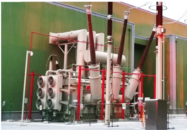
Fig. 2. Electrical transformer installed in \pm 800 kV Zhalute Converter Substation in Inner Mongolia, China.
