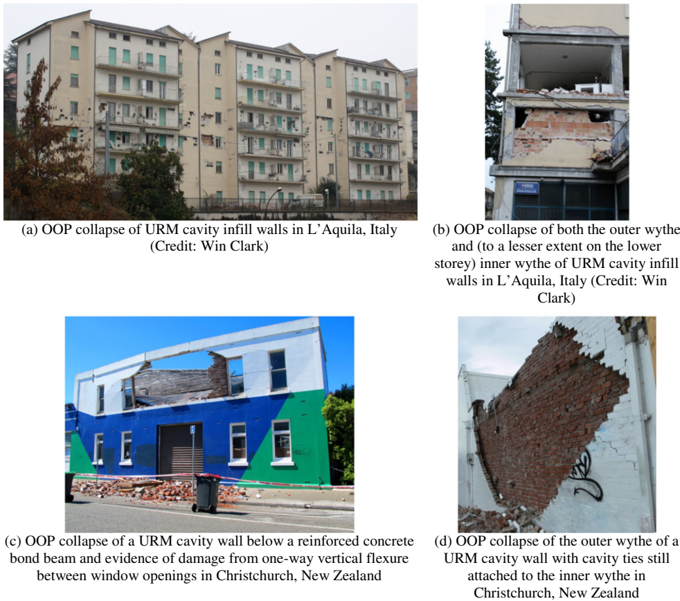
Fig. 1. Examples of OOP collapses of URM cavity walls in earthquakes.
