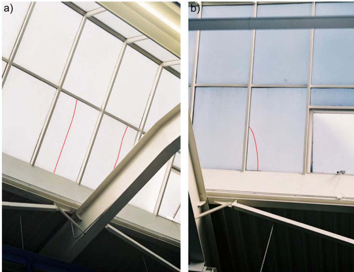
Fig. 2. Cracks in skylight panes: (a) vertical, (b) oblique.
