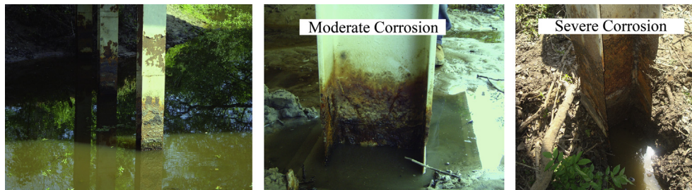
Fig. 1. Deterioration of steel bridge piles.
