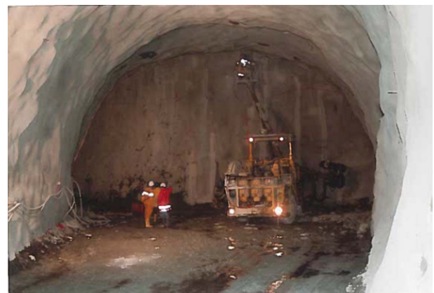
Fig. 2. Irregular tunnel contour after D&B; shotcrete for the first phase support is smoothing asperities and over excavation, but nominal profile is not obtained yet. Suggested D = 0.7 . (Anonymous).
