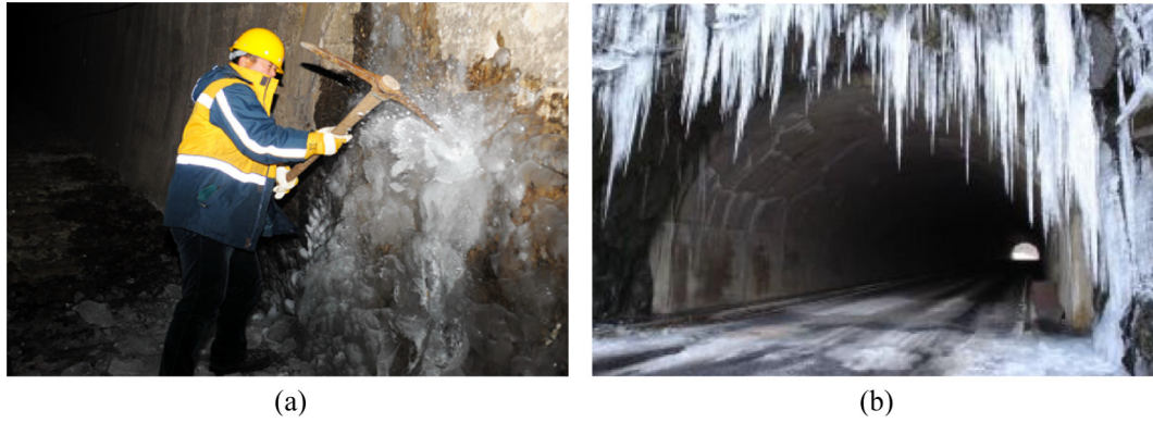
Fig. 1. Frost damages in cold region tunnels (Chen, 2004).
