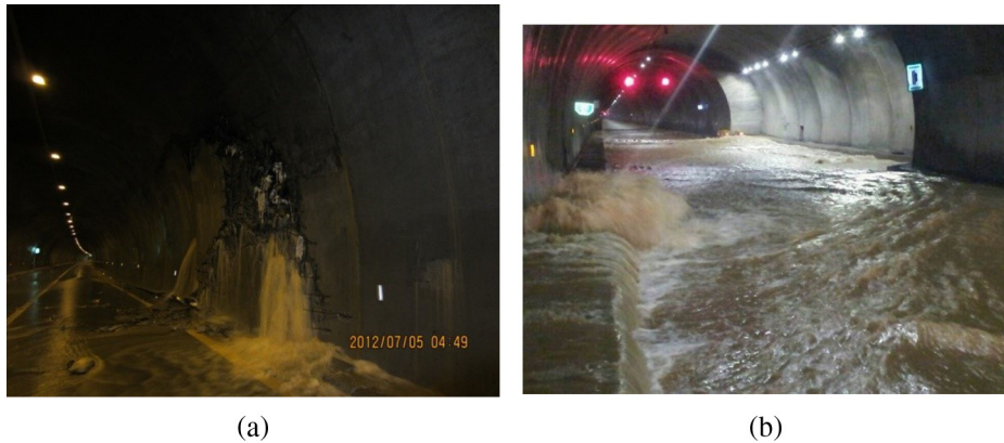
Fig. 1. Liner failure under high external water pressure in Chongqing, China (a) failure at the side wall, (b) failure at the knee.
