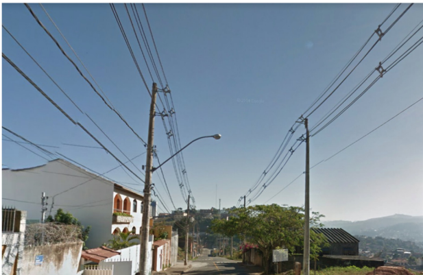
Fig. 1. Two feeders on the same pole - Real DS.
