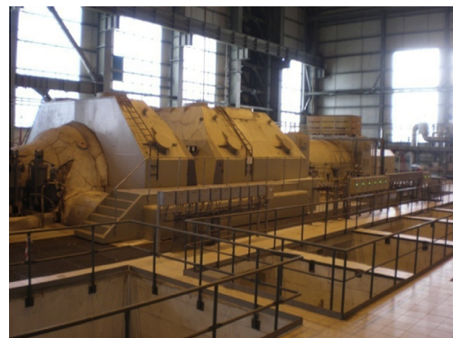
Fig. 3. Turbine and electric generator.
