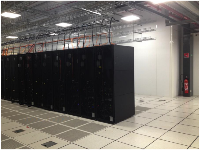
Fig. 1. Data center in Nokia, Lannion.
