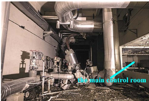
Fig. 1. Scene of steam pipeline explosion (Xinhua Net, 2016).
