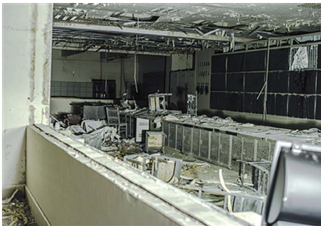
Fig. 2. Scene of the main control room after explosion (Xinhua Net, 2016).
