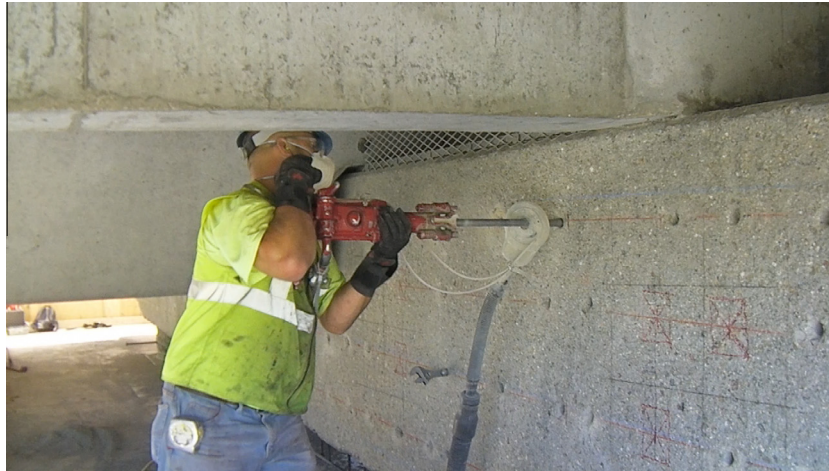
Fig. 1. Usual method for drilling with a 36 lb pneumatic rock drill to drill hundreds of holes for structural upgrade to concrete columns supporting train tracks.
