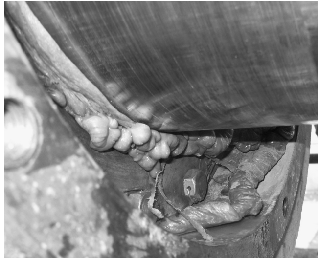
Fig. 1. Melted polymer – the result of an overheated stern tube bearing caused by a cooling system breakdown; shaft diameter 350 mm.
