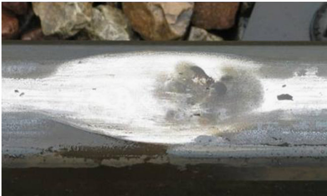
Fig. 1. Well-developed form of a squat defect.
