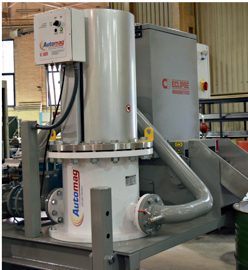
Eclipse Magnetics' Auto-Mag 12 Skid installed at OSL Cutting Technologies, a Sheffield tool manufacturer. Shown here is the cutting and grinding processes using light honing oil.
