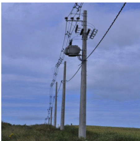
Fig. 1. Distribution line located in a rural area in an open field and crossing grazing lands.
