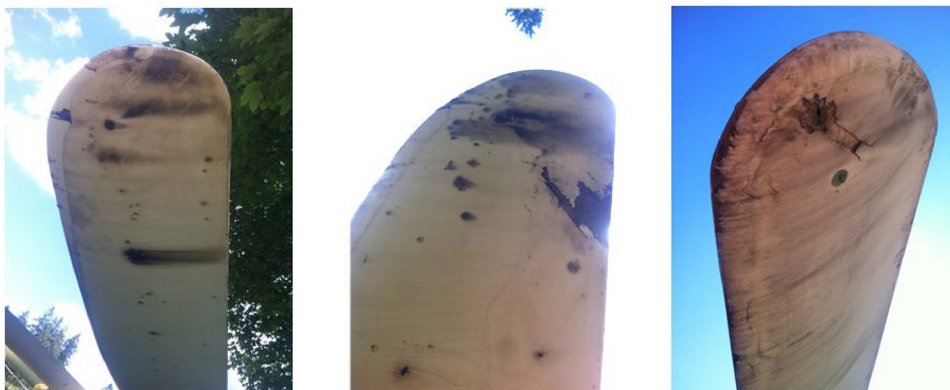
Fig. 2. Damages in wind turbine 6 (WT6) and wind turbine 8 (WT8) caused by lightning.
