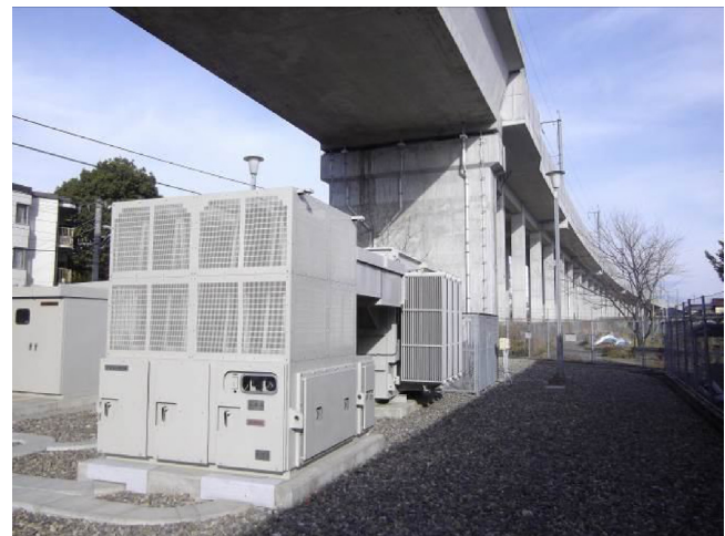
Fig. 2. Installation condition of rectifier.
