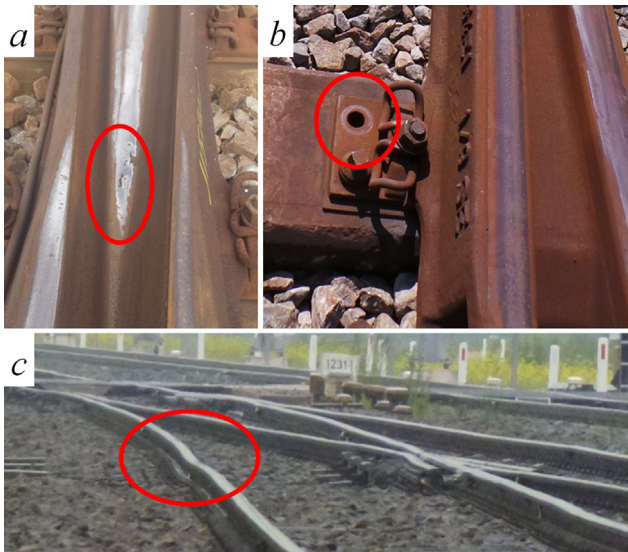
Fig. 1.1. Typical problems in railway crossings: Cracks in crossing nose (a), broken clips (b) and ballast settlement (c).
