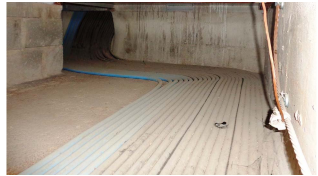
Fig. 1. Arrangement of cables installed in a cement plant.
