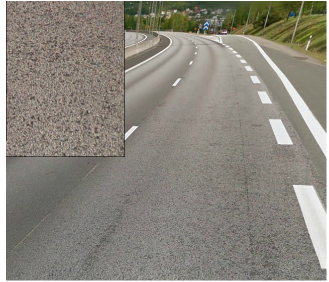
Fig. 2. Inhomogeneous porous pavement due to uneven and excessive wear (and close-up of the wearing course).
