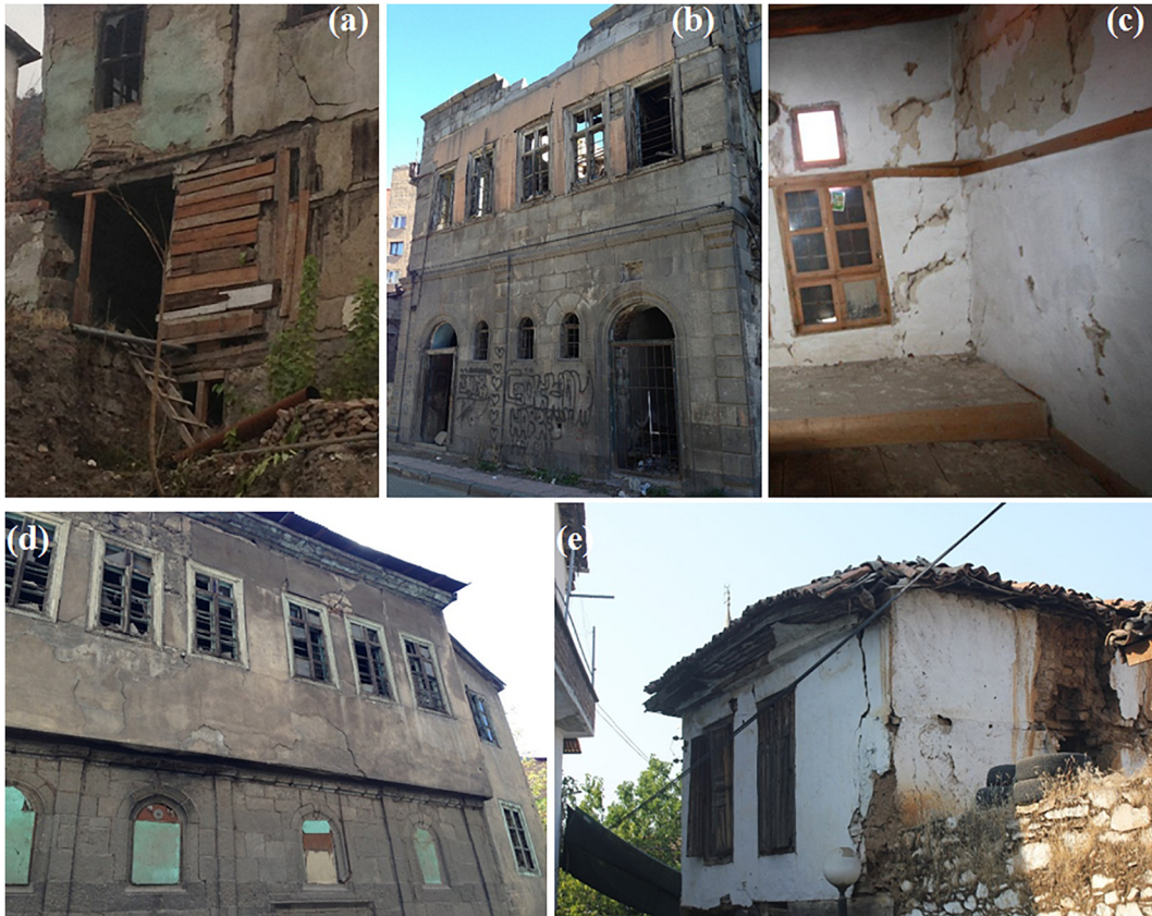
Fig. 1. Typical structural failures of the URM buildings in Turkey after earthquakes (a) Partial collapse in stone masonry walls of the ground floor, (b) Wall-diaphragm tension tie failure, (c) Spalling of masonry unit faceshells and vertical cracking at toe regions, (d) Spandrel joint sliding problem, (e) Vertical cracks at the corners of the masonry wall.
