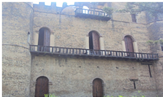
Fig. 2. Buildings in deplorable state.
