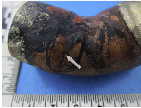
Fig. 1. General view of cracked fitting.
