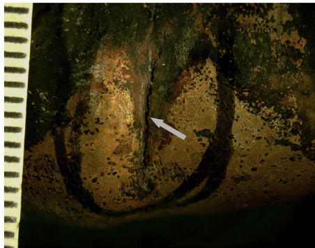
Fig. 2. Magnified view of crack in the external surface of the fitting.
