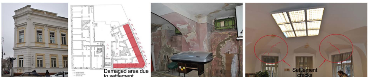
Fig. 2. Severe damages by heavy rain and terrain settlement at a heritage building in Arad, Romania.
