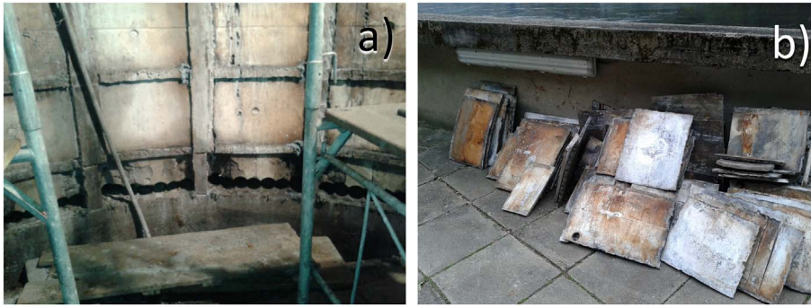
Fig. 1. (a) replacement of draft tube, (b) individual sheets after removing from the draft tube.
