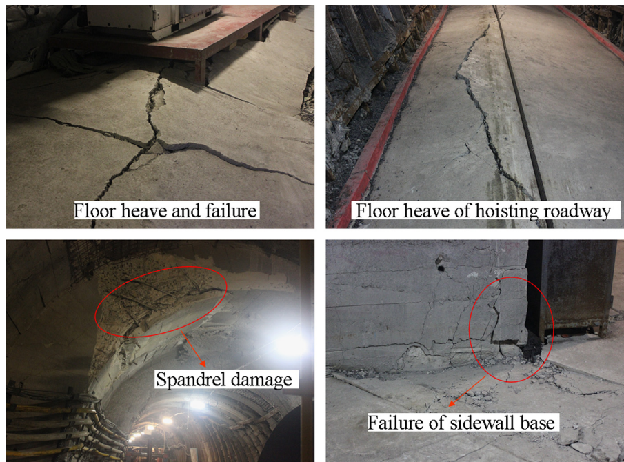
Fig. 2. Serious floor heave and deformation of the winch room of South wing 11-2 in Gubei coal mine.
