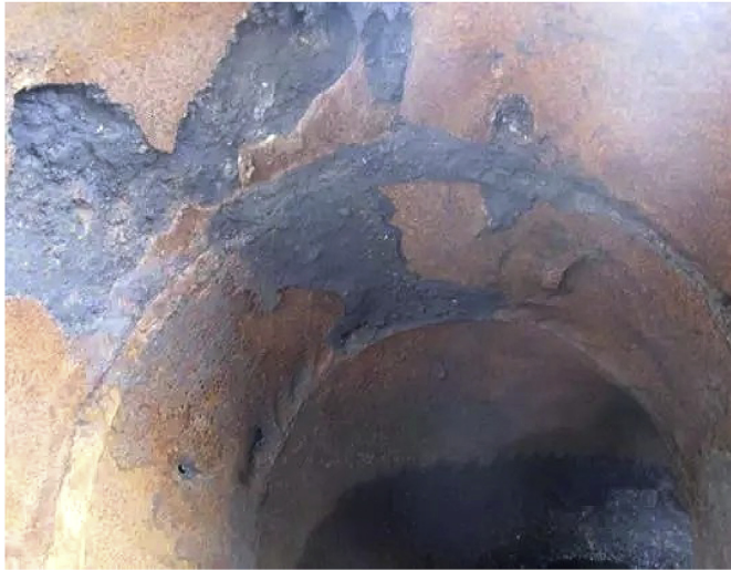
Fig. 1. Erosion on the inner wall of an elbow.
