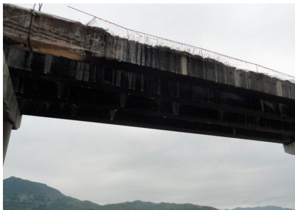
Fig. 1 Fire-damaged PC box girder
