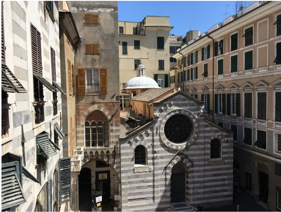
Fig. 1. St. Matteo Abbey in Genoa's old town. The Abbey is surrounded by the houses of the old town, which is also why it is difficult to see its walls and understand the complexity of its humidity problems. In addition to a significant problem of damp rising from the ground—which the present contribution deals with—there are also issues with condensation and infiltration from above. These issues with condensation and infiltration are also linked to a small private terrace above the covering of the left aisle, which complicates the drainage of rainwater.
