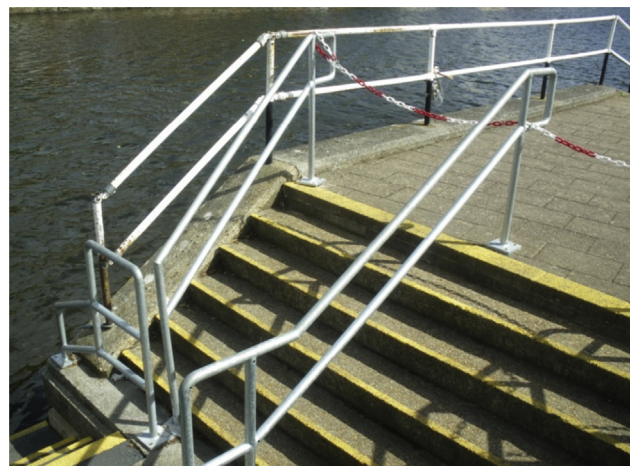
Fig. 2. Changes made to steps following the incident.
