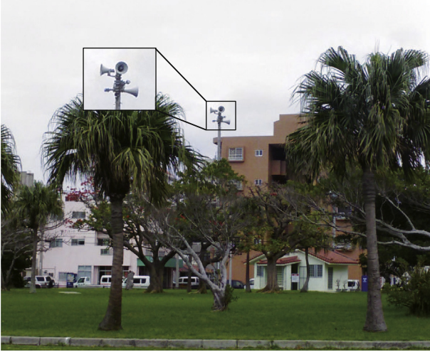
Fig. 1. Outdoor loudspeaker of a public address system for emergency use.
