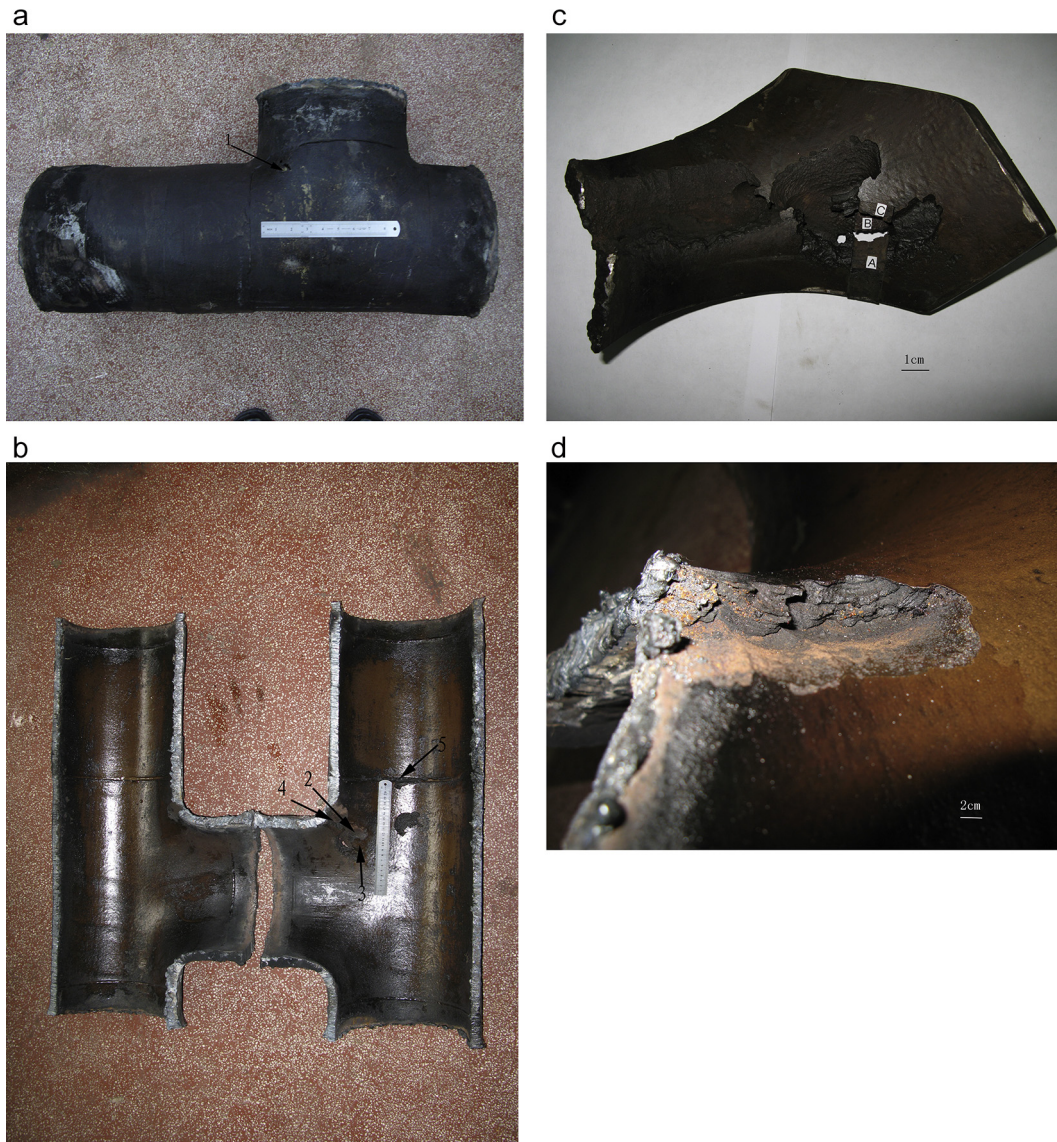
Fig. 1. Interior and exterior of the perforated tee pipe. (a) Exterior; (b) interior; (c) interior of the corroded cavity; (d) interior of location "3" in Fig. 1 (b).
