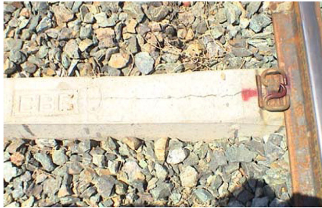
Fig. 1. The longitudinal damage in the concrete sleeper [3].
