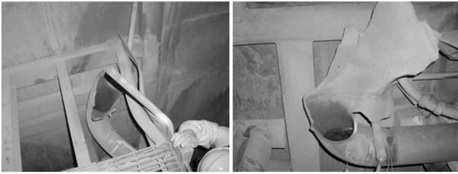
Fig. 1. Pipe rupture due to internal hydrogen-oxygen detonation at Hamaoka NPP [6].
