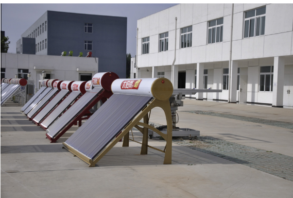
Fig. 1. Water-in-glass evacuated tube solar water heater.
