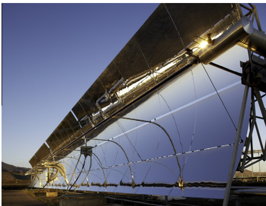
Fig. 1. View of one parabolic-trough solar collector of the DISS test facility.
