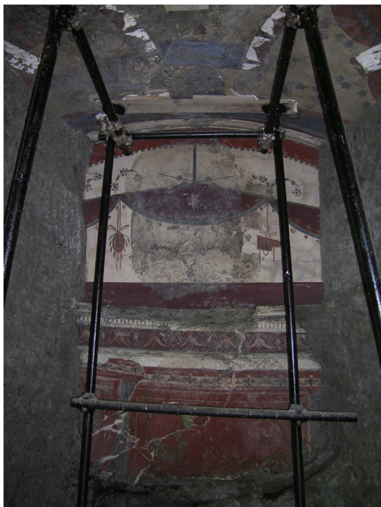
Fig. 1. A partial view of the Northern room in the Basis Villa with deterioration phenomena on the vault (little white squares in the upper corners and Lotus flowers on the top).
