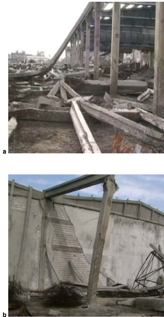
Fig. 1. General view of plant after fire: (a) collapsed structural members and (b) deformed column and beam.
