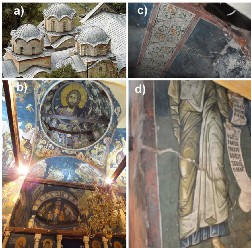
Fig. 1. a) Image of the Peć Patriarchate complex, Serbia; b) dome of the Church Hodegetria; c) detail of a wall painting with the efflorescence; d) detail of a wall painting with craquelures.
