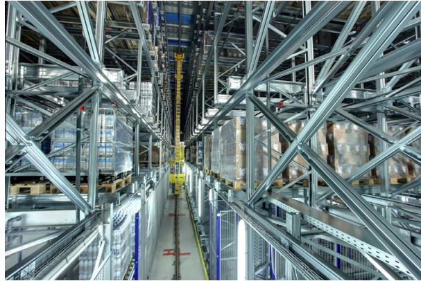
Fig. 1. Typical installation of a high rack with monorail shelf feeder. Source: http://group.emmi.com .
